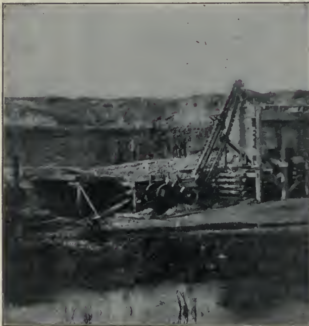
Arrangement of Crushing Equipment—Oxford County—Crusher below floor of quarry; limestone fed to hopper over crusher, and crushed material elevated to revolving screen and storage bin.
